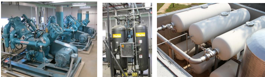
Figure 2 – High-pressure air supply system including compressors (left), dryers (middle), and storage tanks (right)
